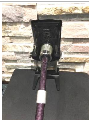
Power Distributor & Wall Receptacle
